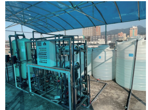
Cleaning wastewater recycling devices
