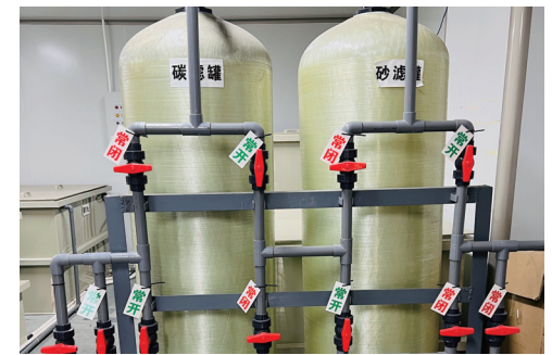
Wastewater recycling facilities
