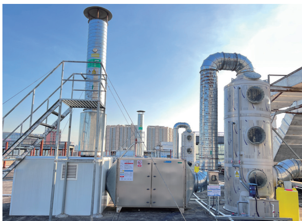
Waste gas treatment facilities
